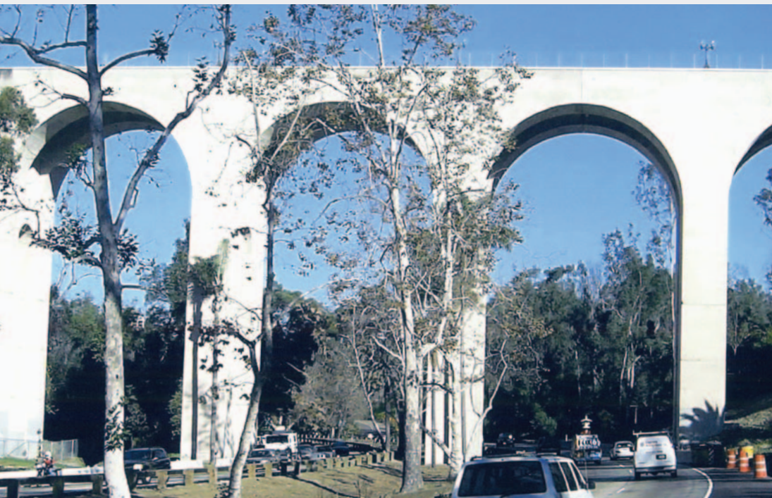
Cabrillo Bridge, San Diego, CA ICRI 2006 Award of Excellence in Historic Restoration
