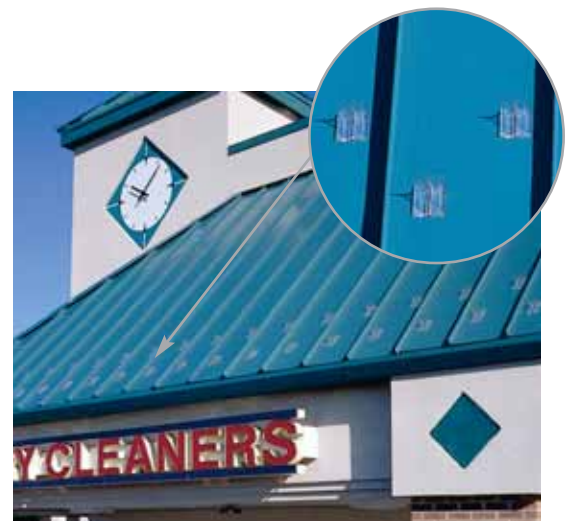
This shopping center features Berger Clear Snow Guards. They are manufactured in a crystal clear polycarbonate to offer superior protection with an out-of-sight look.
