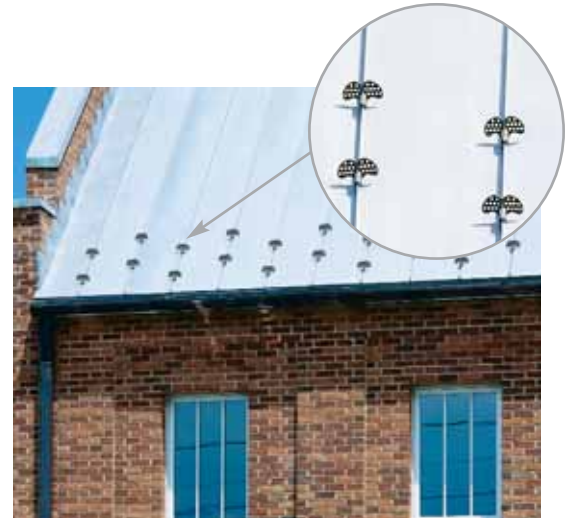
The roof on this church details the use of Berger cast aluminum "RT Snow Guards".
