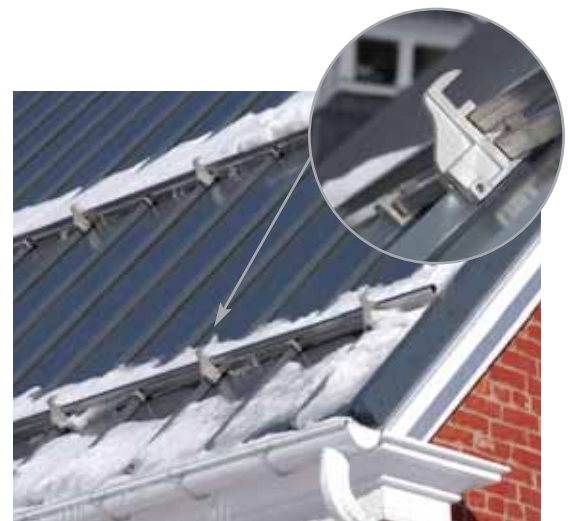
The roof on this church details the use of the Berger "F-Rail"™ Snow Retention System
