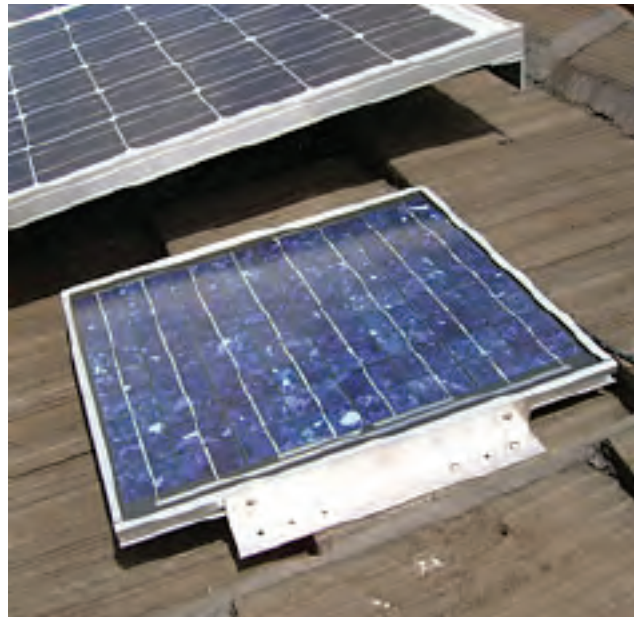
remote solar panel installed on roof
