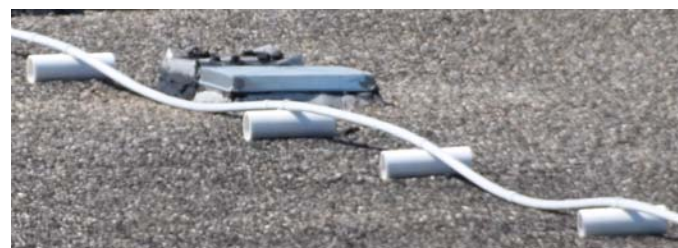
Picture 3: Inappropriately supported PVC pipe.
