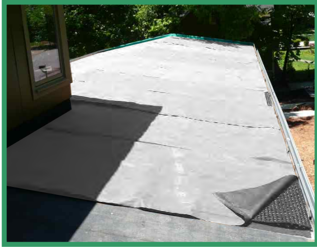
Residential Greenroof, Atlanta, GA (Photo Courtesy David Butler Architects & Thomas Nichols, RLA)
