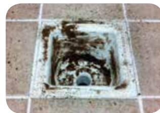
Rusted floor sink
