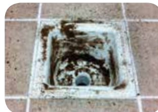
Rusted floor sink
